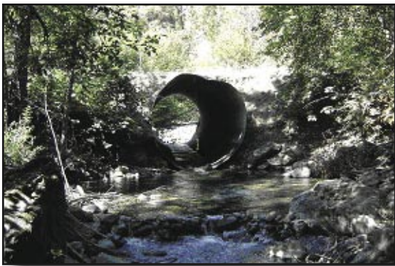
High valasity culvert barrier blocking fish passage to four miles of habitat on Fort Goff Creek
