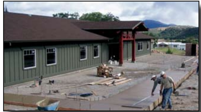
Subcontractors working on walkway in front of new Yreka KTHA Building- photo by Fred Burcell, KTOC Construction Manager
